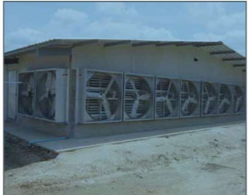
An Example of Power Ventilation
