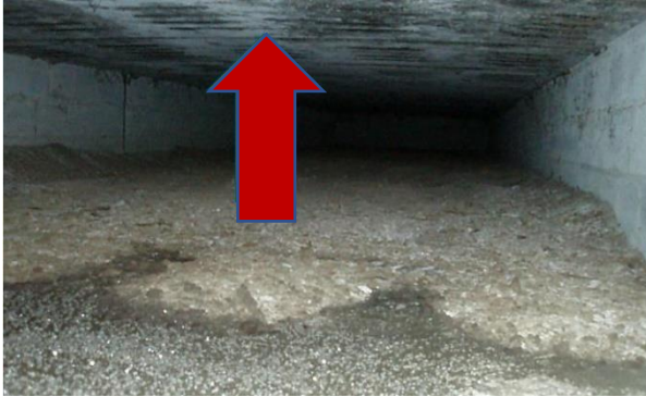
Figure 3 - Underground duct with loose material and CIPC deposits.
